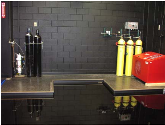
(a) A view of the compressed air filling system.
